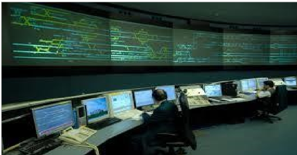
Figure 22-4 CTC Control Centre at Tundla
