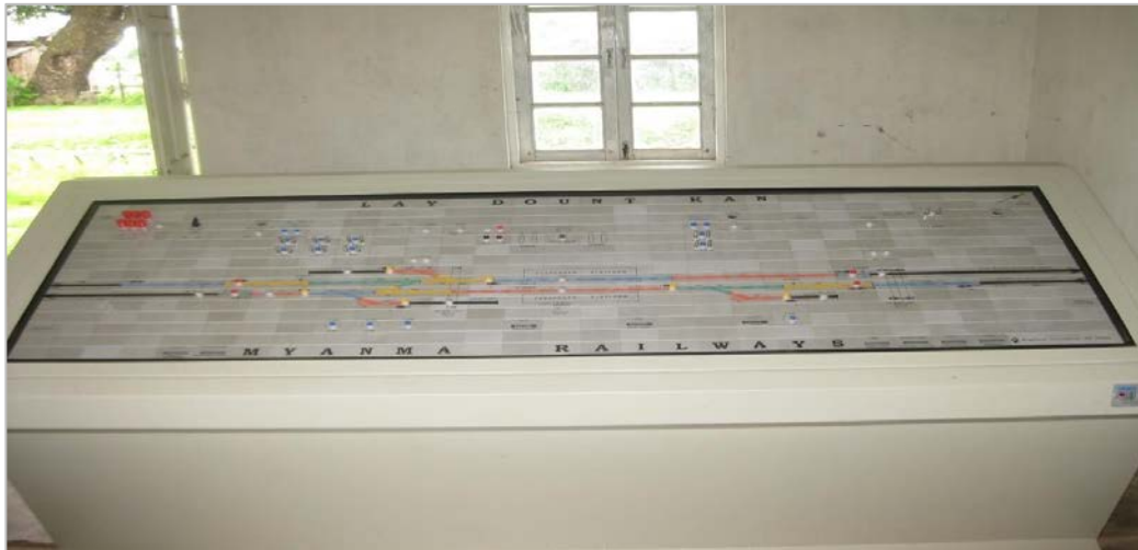
Figure 22-2 Signaling Panel at IR station
