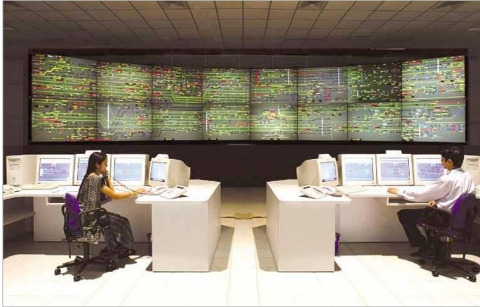
Figure 22-5 Train Management System at Mumbai
