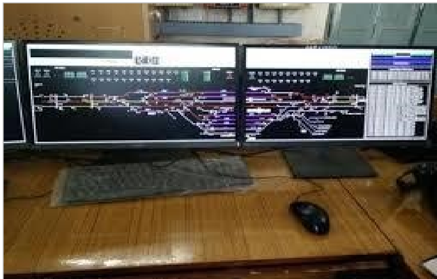
Figure 22-3 VDU and Key Board based Station Control at EI station
