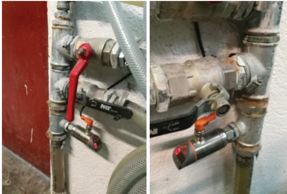
Figure 7.25 Sensors installed in the refrigeration circuit.
