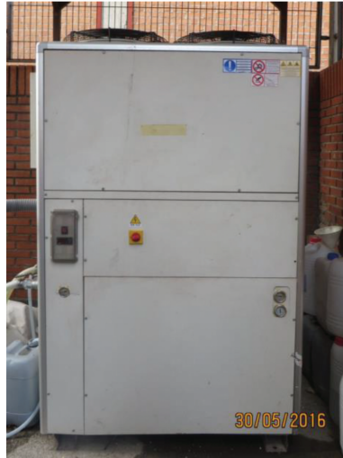
Figure 7.22 Cooling system from injection chamber.
