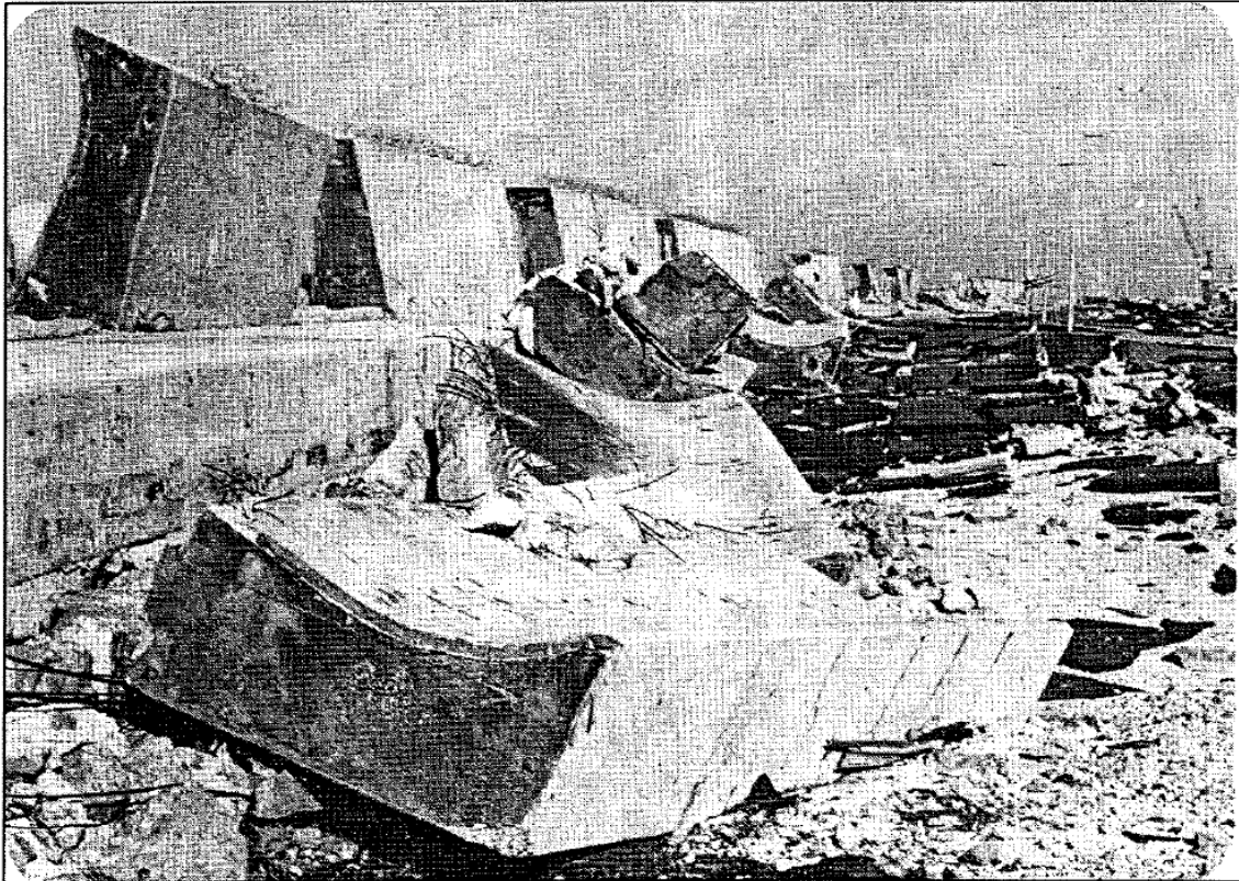
Broken crown wall sections on the Tripoli Harbor NW breakwater after a storm in 1981 (Pedersen, 1996)
