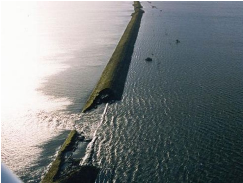
Juvre Dike breached after the storm surge in 1999 (www.kyst.dk, 2013)
