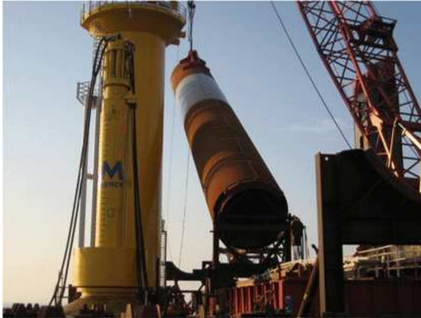
Figure 1: Monopile foundation being loaded on board a vessel. The yellow pillar at the rear is a transition piece. www.dongenergy.com
