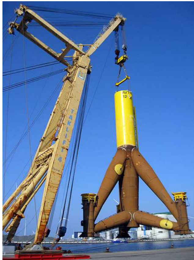
Figure 4: Tripod foundation for a 5 MW wind turbine at the Alpha Ventus offshore wind farm, Germany. www.owt.de .
