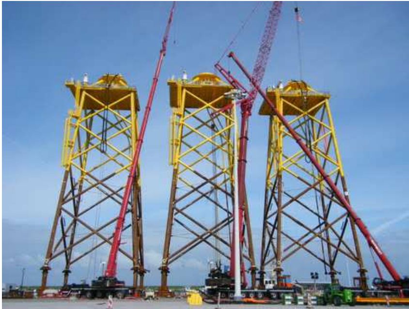
Figure 5: Jacket foundations for the 5 MW wind turbines at the Alpha Ventus offshore wind farm, Germany. www.panoramio.com .
