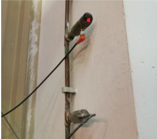
Figure 7.34 Pressure and temperature sensor installed in the compressed air circuit.
