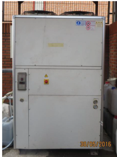
Figure 7.22 Cooling system from injection chamber.
