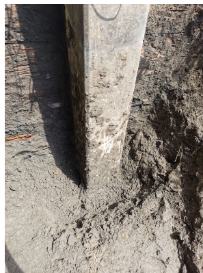
(b) Exposed pile scour detailed view (D2)
