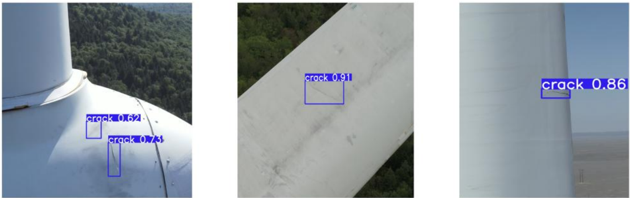
Fig. 4 Samples of predicted cracks on wind turbine using YOLOv8.
