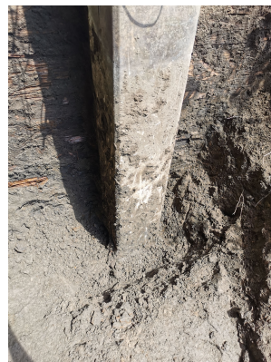
(b) Exposed pile scour detailed view (D2)
