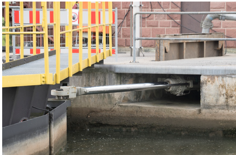
Figure 1.1: Hydraulic cylinder for moving a lock gate
