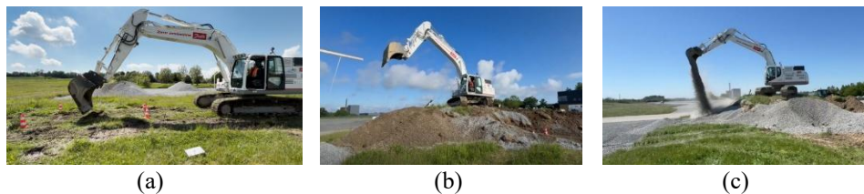
Figure 3.1. (a) JCMAS Air-Grading, (b) Air-Dig and Dump, (c) Real Dig and Dump
