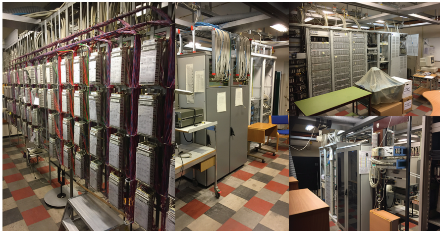
Figure 9.4 Digital exchange for ship-to-shore radio anno 1999 in Denmark [6].
