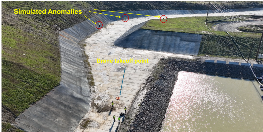
Fig. 3 Simulated anomaly locations of the spillway.
