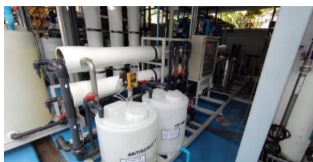
Figure 7 Ultrafiltration and Reverse Osmosis System
