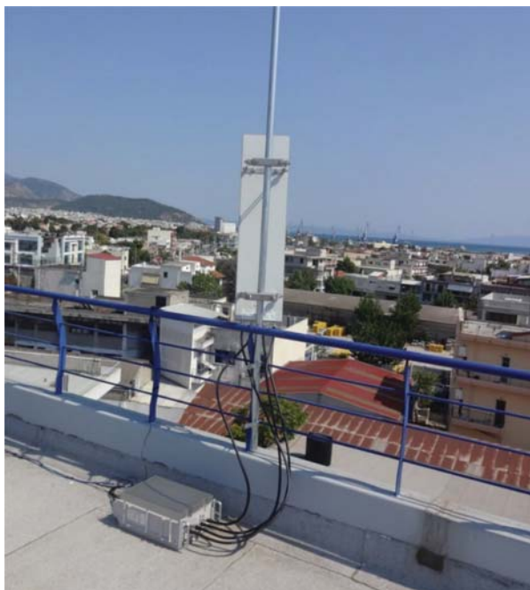
Figure 12.6 WiMAX/LTE Base Station in NITOS testbed.
